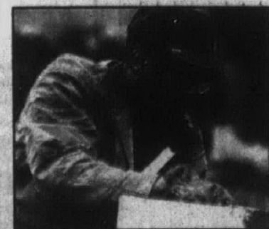
Heavy load: Aaron Hill of Canton was part of the crew which passed concrete blocks to volunteer masons building the foundation wall.
