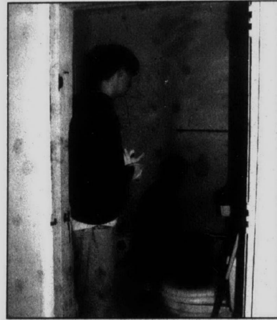
Making repairs: Catholic Central High School student Ryan Wilmering offers a few "pointers" to his father, Richard, while preparing the bathroom for a fresh coat of paint and new lighting.
