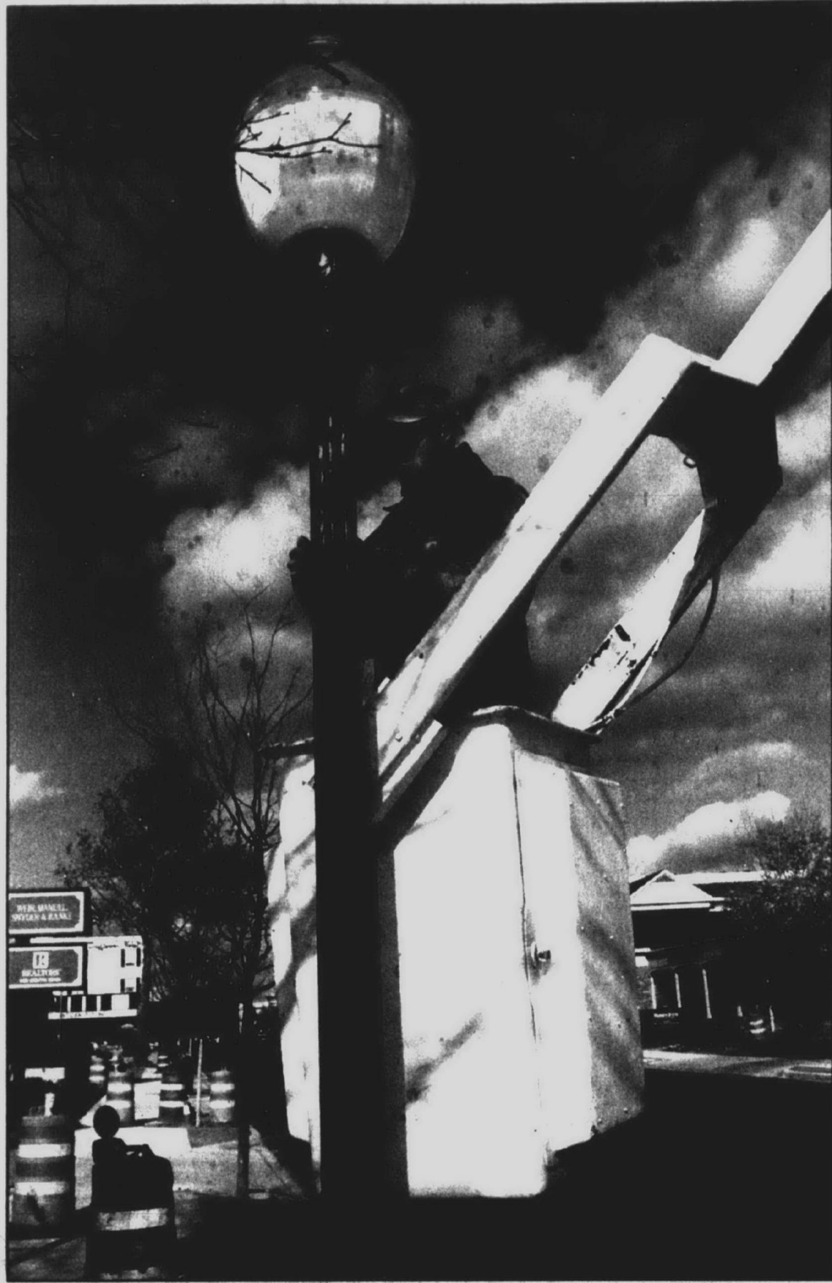
Street work: Mark Leid, an electrician working on the downtown streetscape project, installs street lamps on Friday afternoon.
