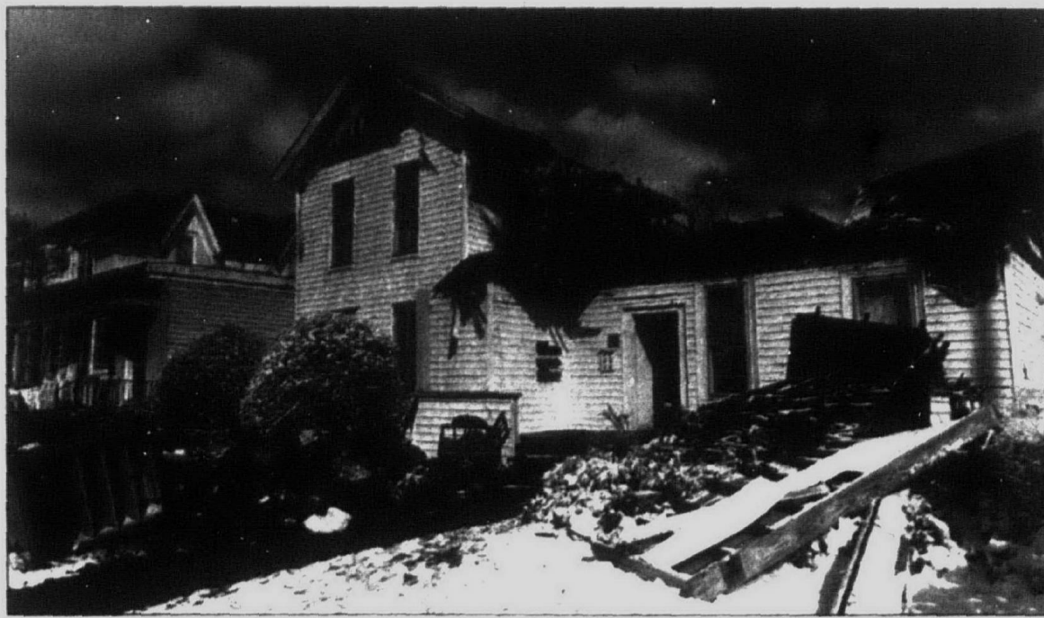
Bill Breesler/Staff Photographer Last look: Severly damaged by fire on Thursday, this apartment building on Penniman was scheduled for demolition Friday.
