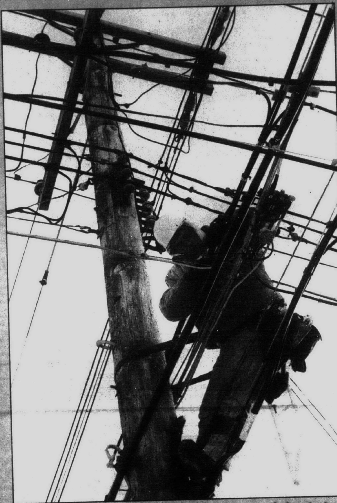
Making it better: Aaron Weisel, a contractor for Continental Cablevision, splices fiber optic cable into the firm's upgraded system.
