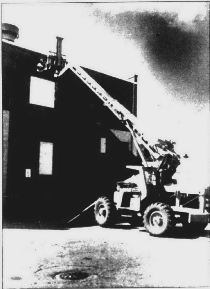
Renovation: Crews worked throughout the summer at Central Middle School, removing asbestos, remodeling offices and lounges, replacing plumbing and electrical equipment, painting and polishing Landsay Walker (above, left) of Lydell and Hart, a Livonia mason contractor, reads Central for the installation of an elevator.
