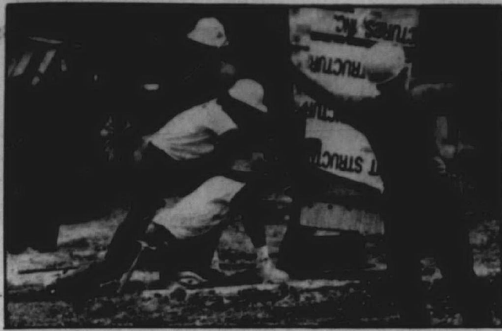
At work: Construction workers at the site concentrate on the task at hand. Worshipers at the Canton congregation hope to have the project completed by February or March of next year.
