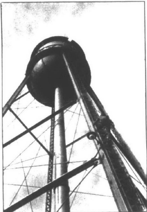
Towering job: Preston Hill of Federal Salvage of Livonia climbs the tower to prepare cables used to pull it down.
