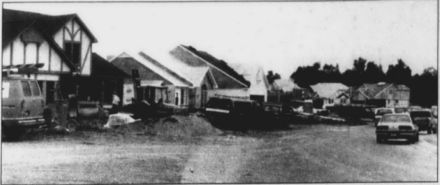
Housing recovery: With interest rates holding at low levels and the economy picking up, builders are optimistic about prospects for 1992 after a good first quarter.
